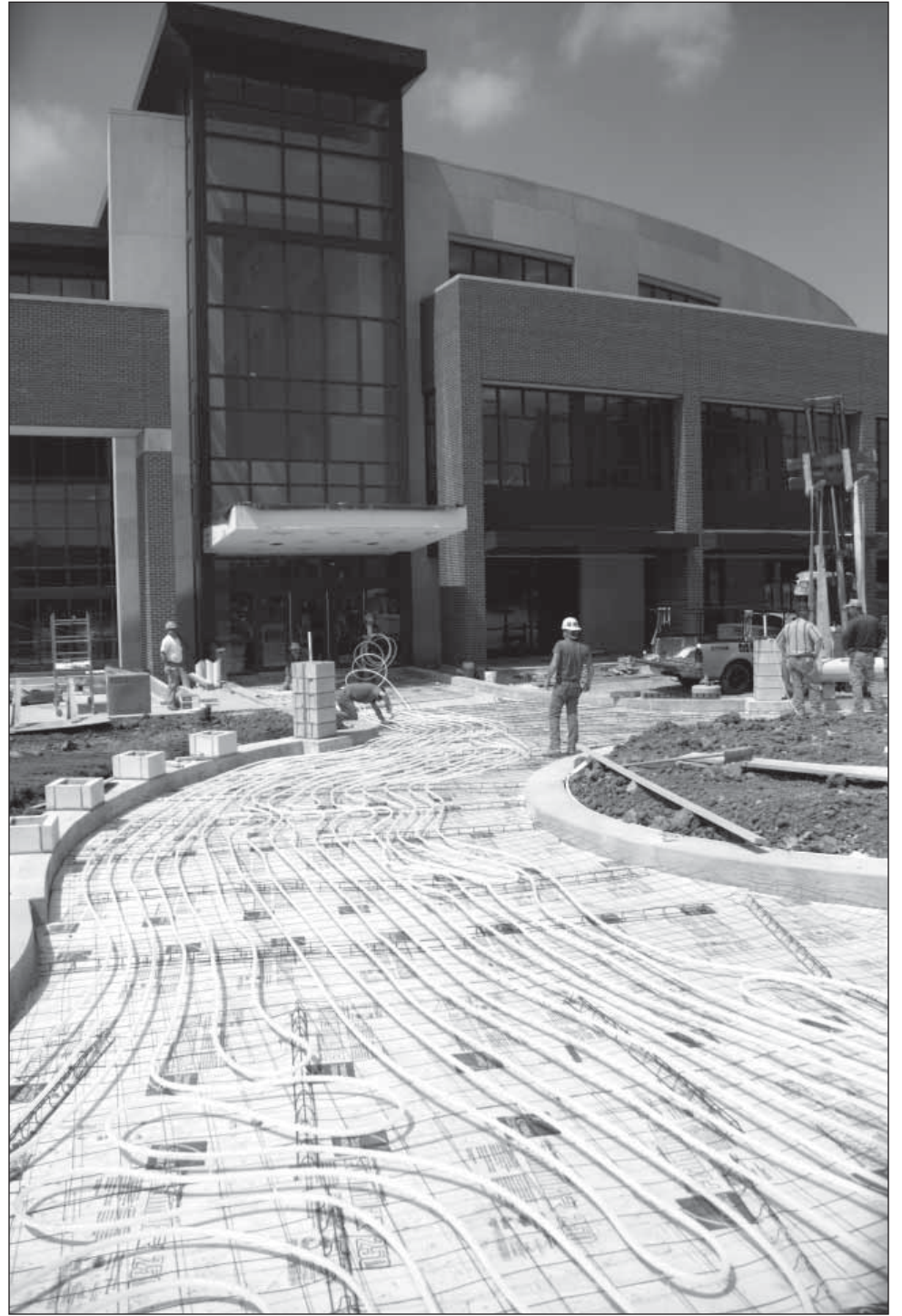
Heated piping runs beneath the entryway to the new Communication and Media Building set to open for the Fall 2007 semester. Photo by Doug Blemker
